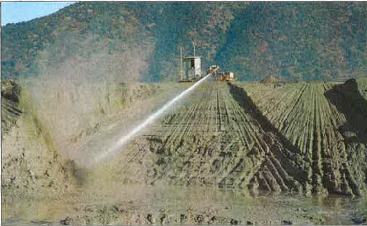
A hydraulic monitor moves old tailings material at Amerigo Resources' MVC processing operation in Chile.
